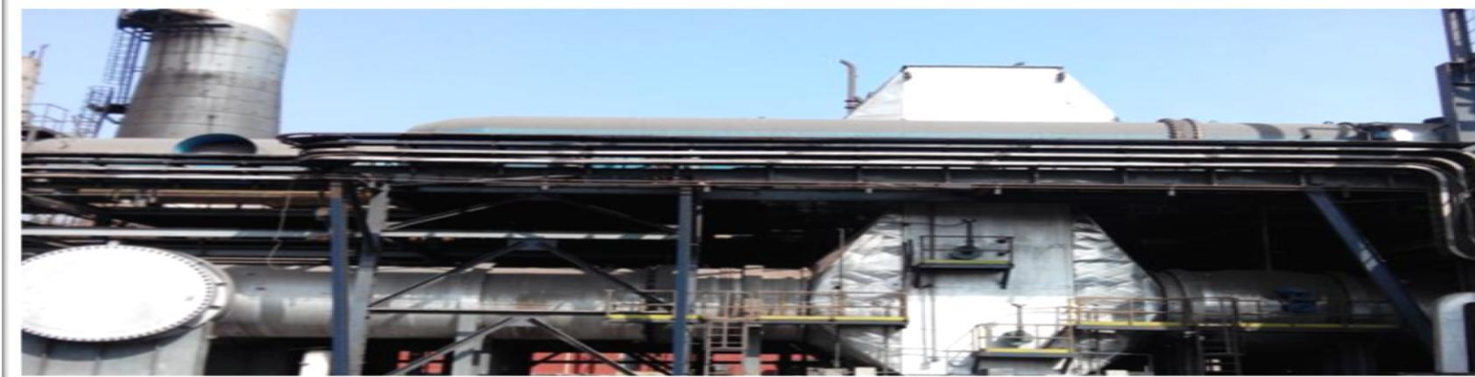
Waste Heat Recovery System at BF-4 in Vijayanagar: Commissioned in Nov 2013
